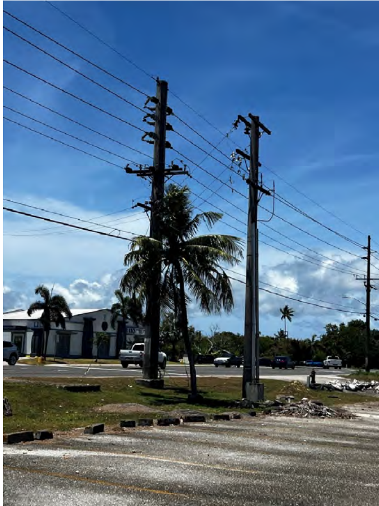
PHOTO #1 - EXISTING CONDUIT RISER ON GPA POLE ALONG ROUTE 10
