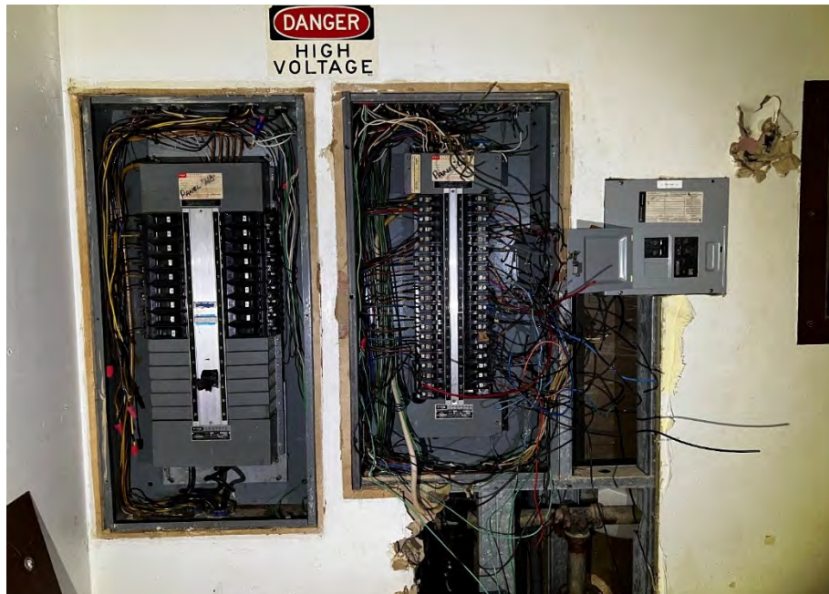
PHOTO #5 – PANELBOARD WHERE FIRE INCIDENT OCCURRED
