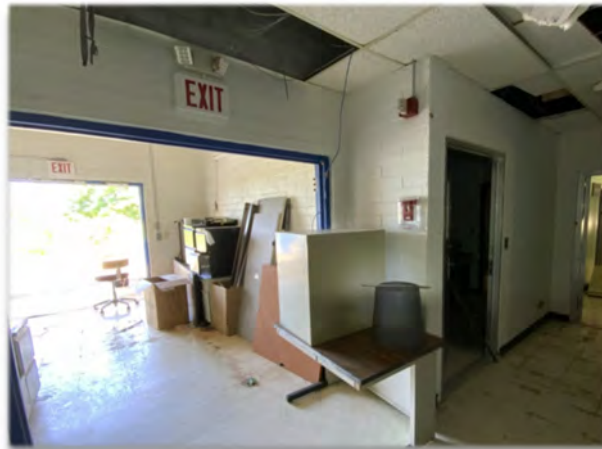
Fig. 7 Stair handrails, no guard rails.
