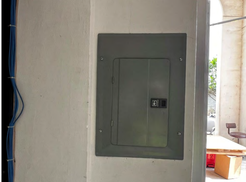
PHOTO #4 – PANELBOARD AT MAIN BUILDING ENTRANCE
