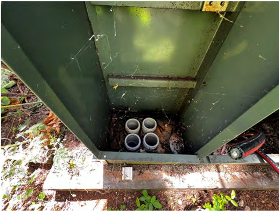
PHOTO #7 – THEFT OF TRANSFORMER PARTS AND WIRING
