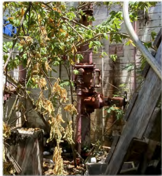
Fig. 1 Closed Fire Sprinkler Riser
