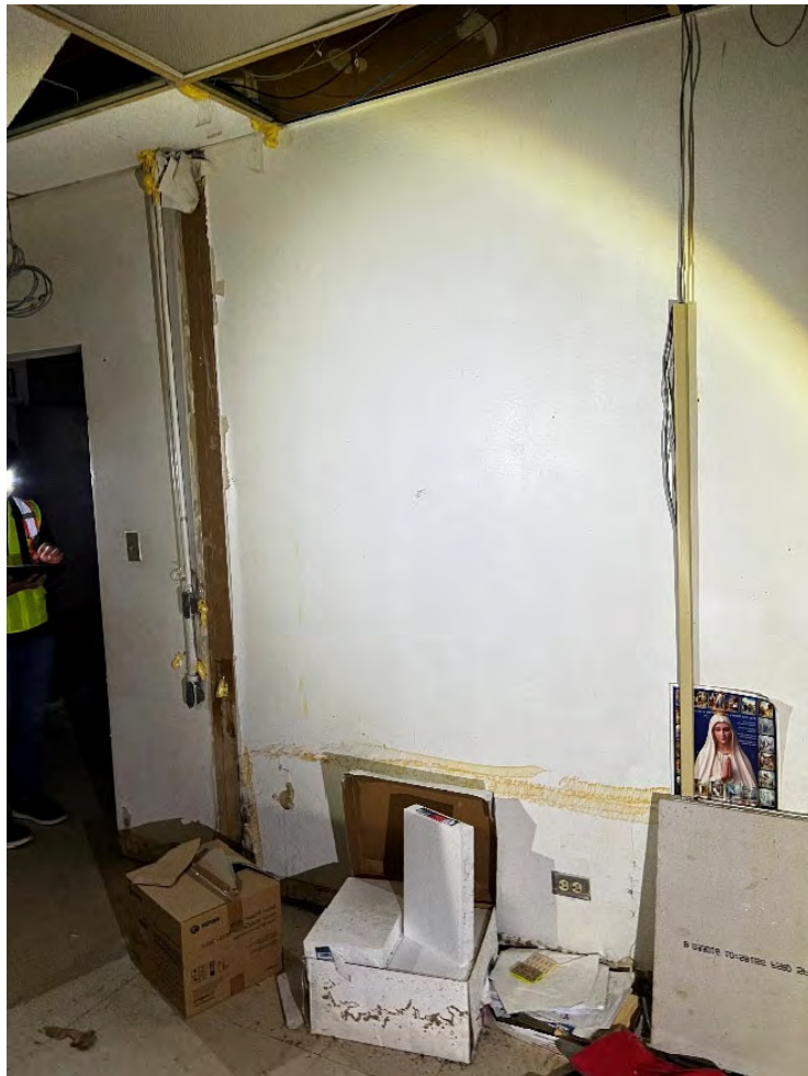
PHOTO #8 – OUTLETS AND SWITCHES, OLD AND CORRODED
