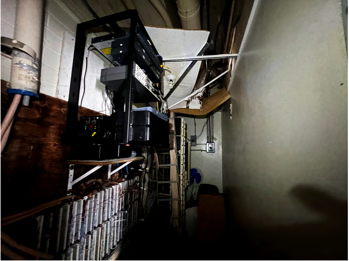
PHOTO #10 - EXISTING TELECOM ROOM
