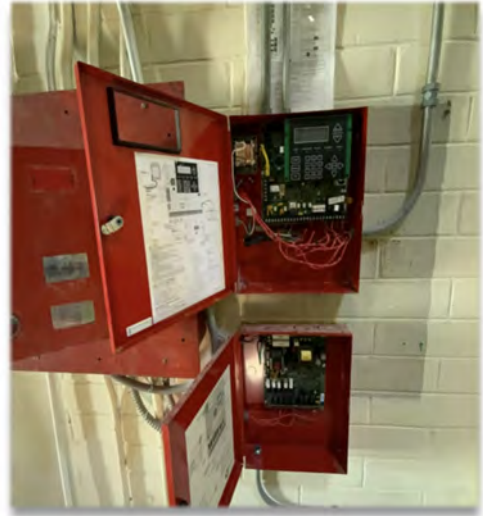
Fig. 3 Silent Knight Fire Alarm Control
