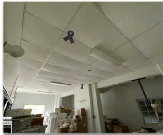
Fig. 2 Room with no sprinkler protection
