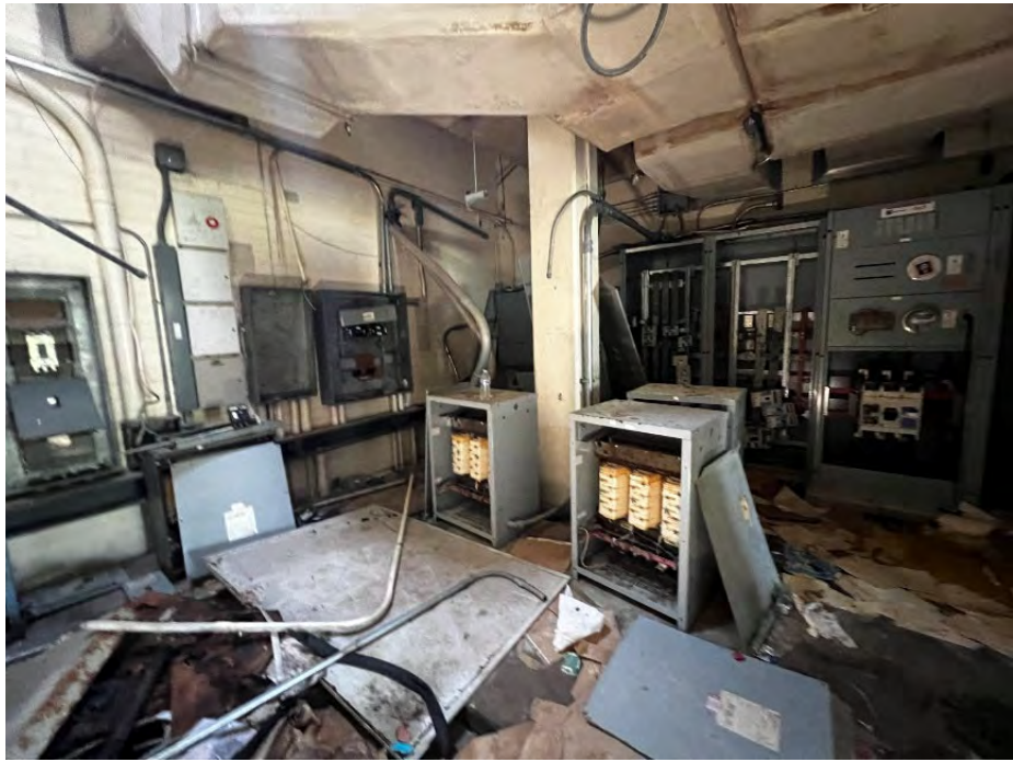
PHOTO #3 – UNUSABLE ELECTRICAL EQUIPMENT, CONDUITS, AND WIRING
