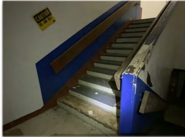
Fig. 6 Stair handrails, no guard rails.
