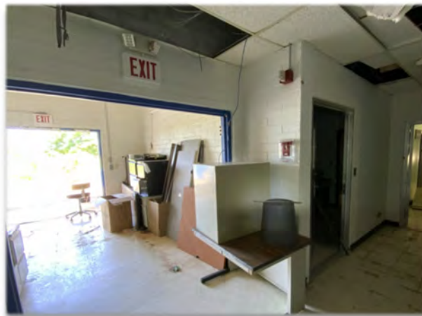
Fig. 7 Stair handrails, no guard rails.
