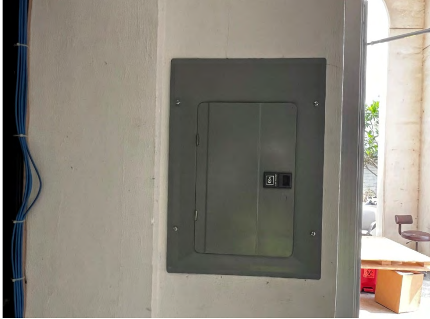
PHOTO #4 – PANELBOARD AT MAIN BUILDING ENTRANCE
