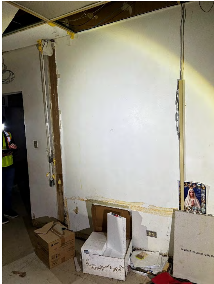
PHOTO #8 – OUTLETS AND SWITCHES, OLD AND CORRODED
