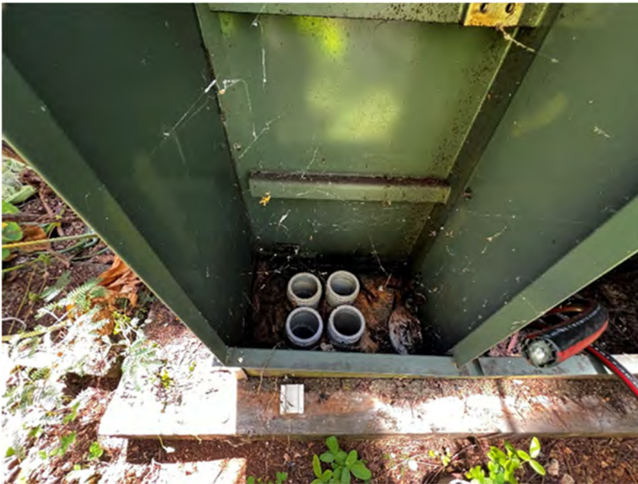
PHOTO #7 – THEFT OF TRANSFORMER PARTS AND WIRING
