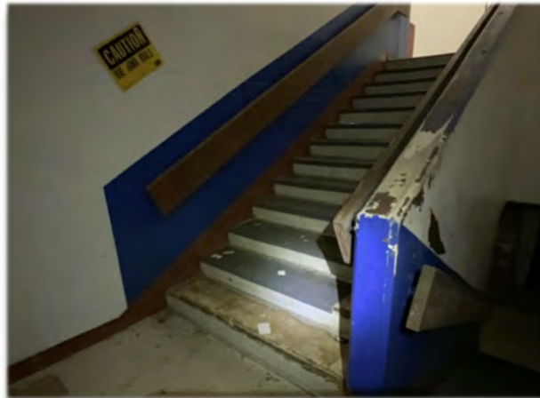
Fig. 6 Stair handrails, no guard rails.
