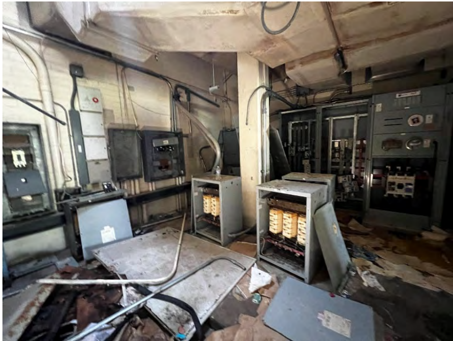
PHOTO #3 – UNUSABLE ELECTRICAL EQUIPMENT, CONDUITS, AND WIRING
