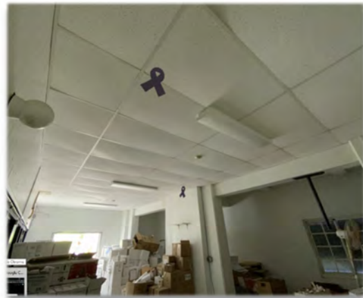
Fig. 2 Room with no sprinkler protection
