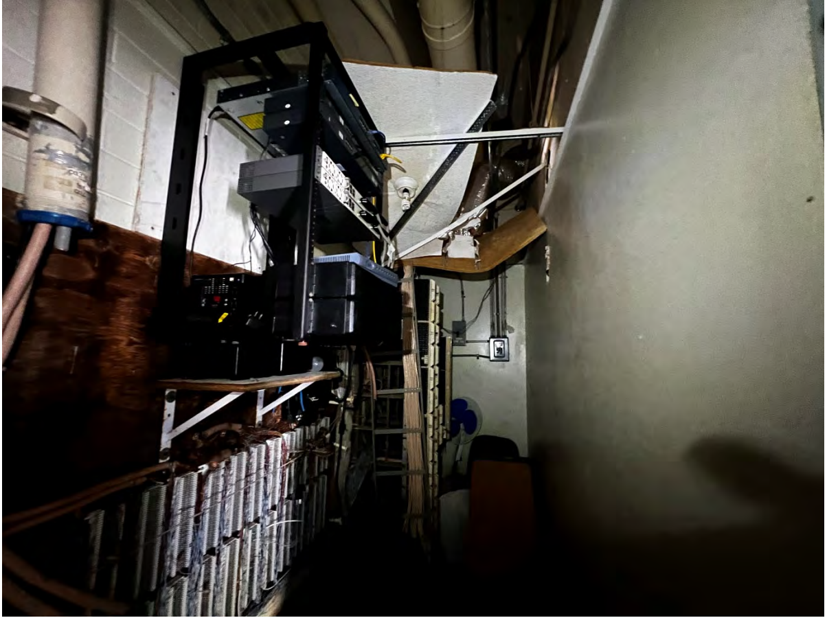
PHOTO #10 - EXISTING TELECOM ROOM
